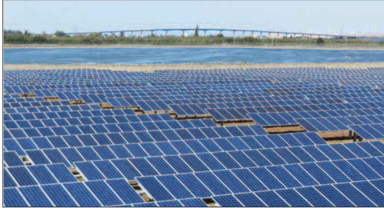
Hundreds of solar panels at the ISD solar energy farm catch some afternoon rays.
