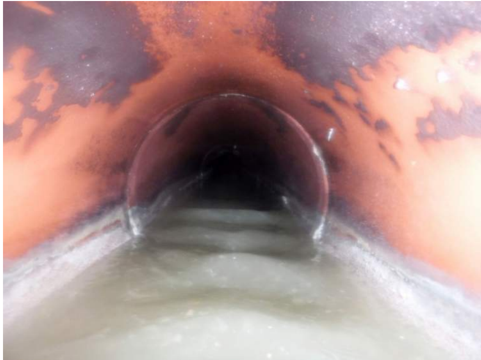
Monitored South Influent Pipe
