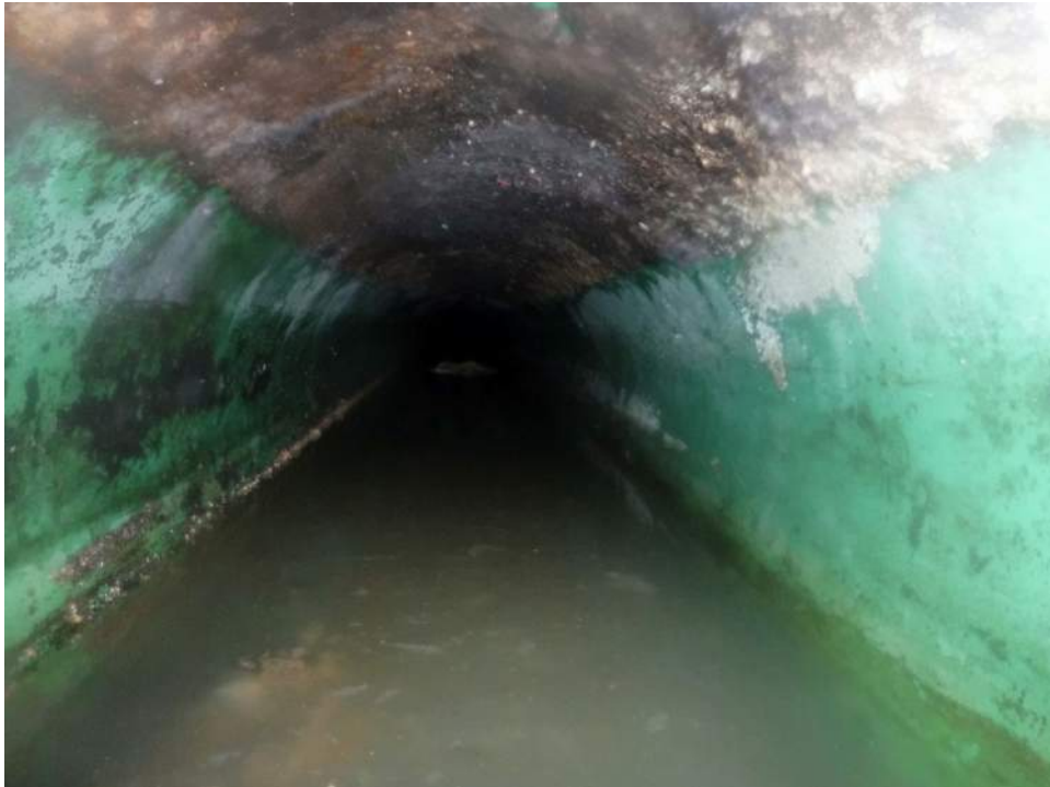
Northwest Effluent Pipe 2
