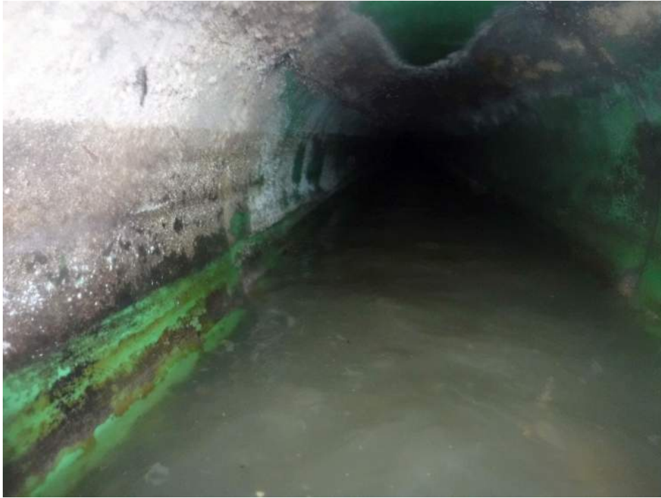
Northwest Effluent Pipe 1
