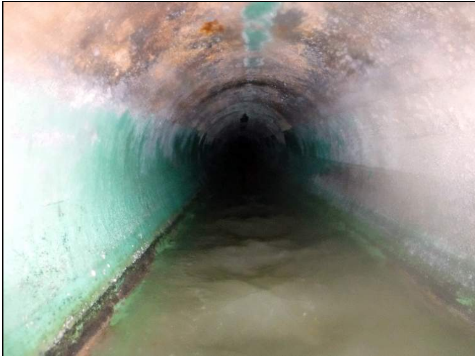
Monitored Southeast Influent Pipe
