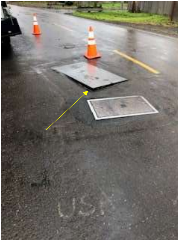
Above: Broken hinge bracket is causing the south east corner of the lid to lift creating a road hazard
