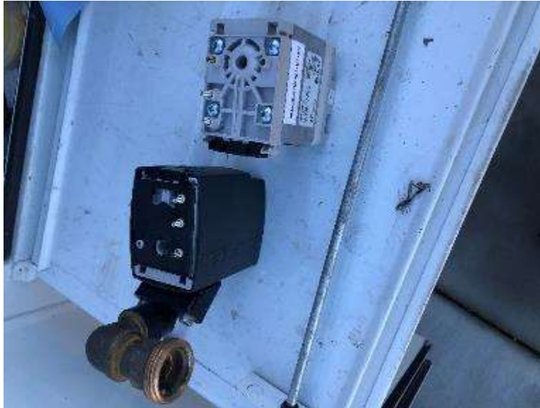
Failed and replacement Auto Drain components
