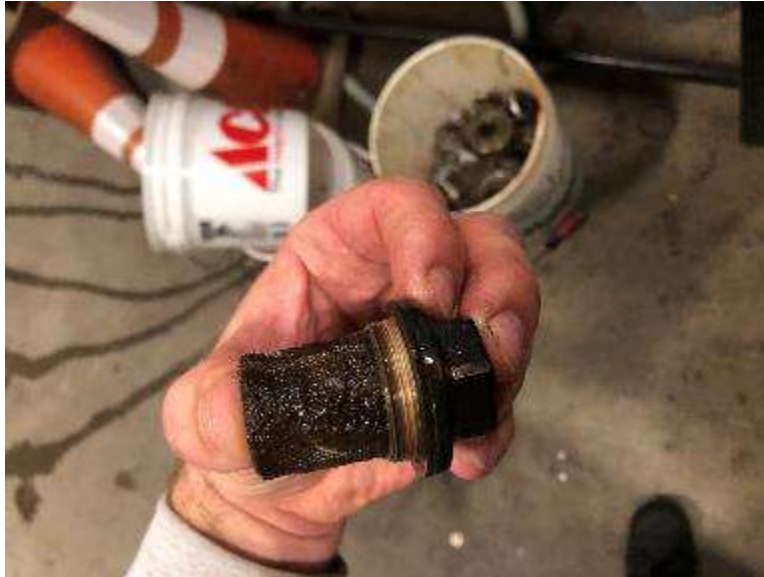
Buildup on PRV Inlet Screen
