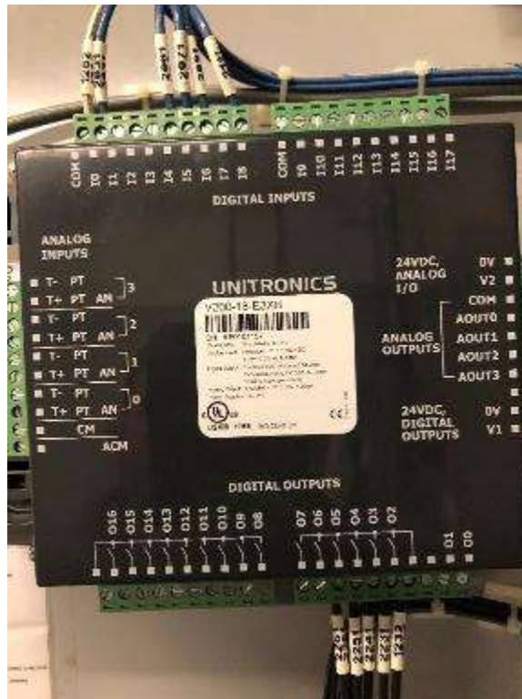
Failed HMI Control Card
