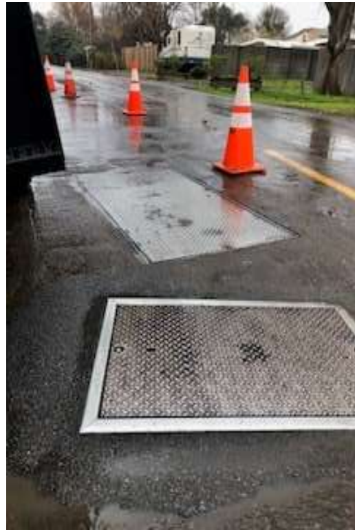
Above: Collections crew temporarily corrected the issue by securing the lid with bolts and backing plates, the lid is scheduled for replacement
