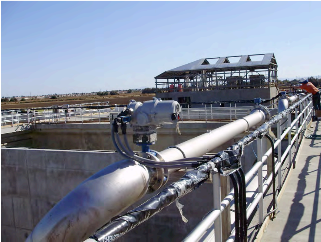
AA Basin Control Valves and Electrical Installation Solids Handling Building Roof Installation in the Background
