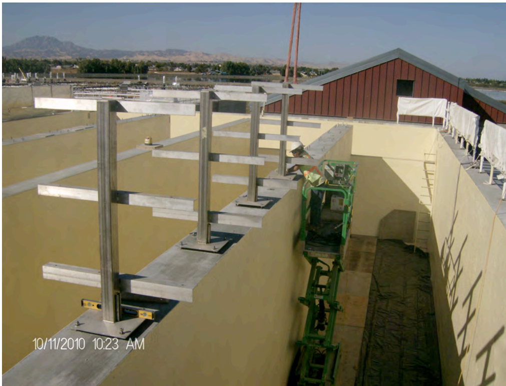
MBR Building: Coating Completed, Pipe Support Installation Chem/Blower Building Siding in the Background
