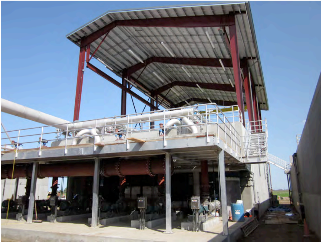
MBR Structure Ready for Startup Activities
