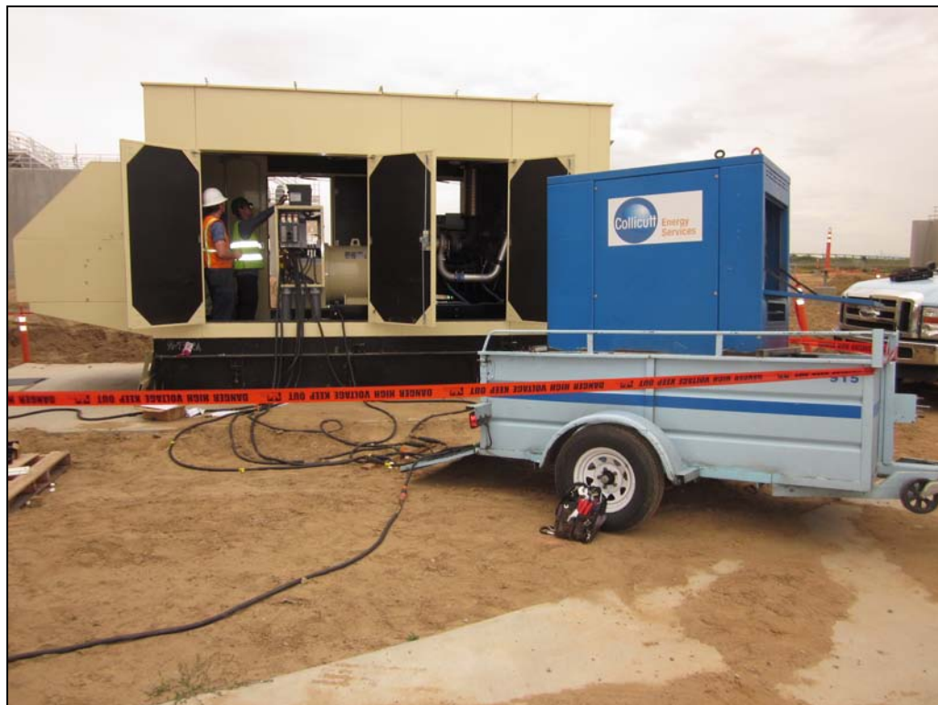
Generator Field Testing
