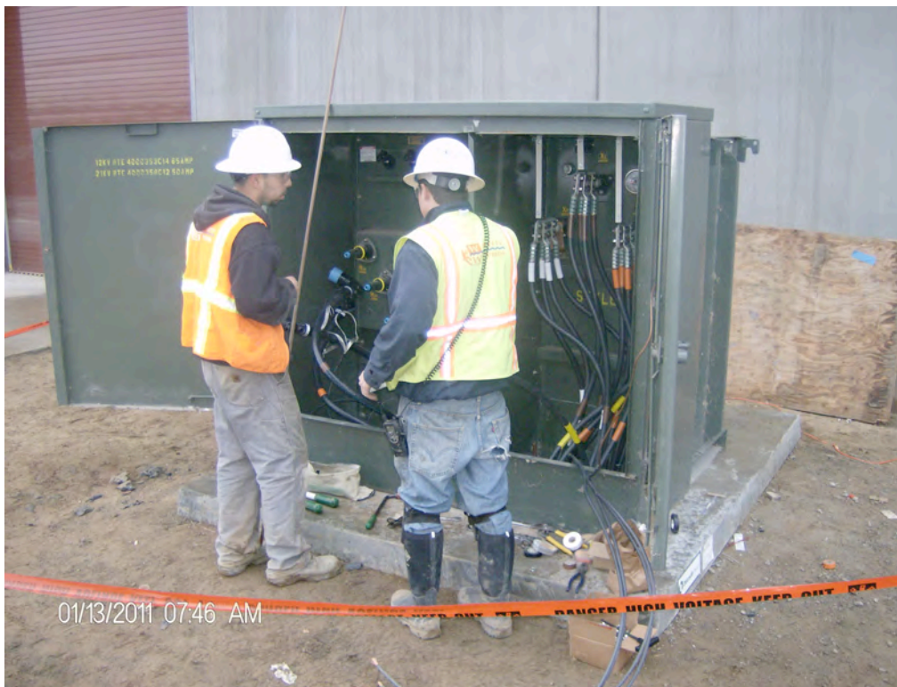
Wire Terminations at the Solids Handling Building Transformer
