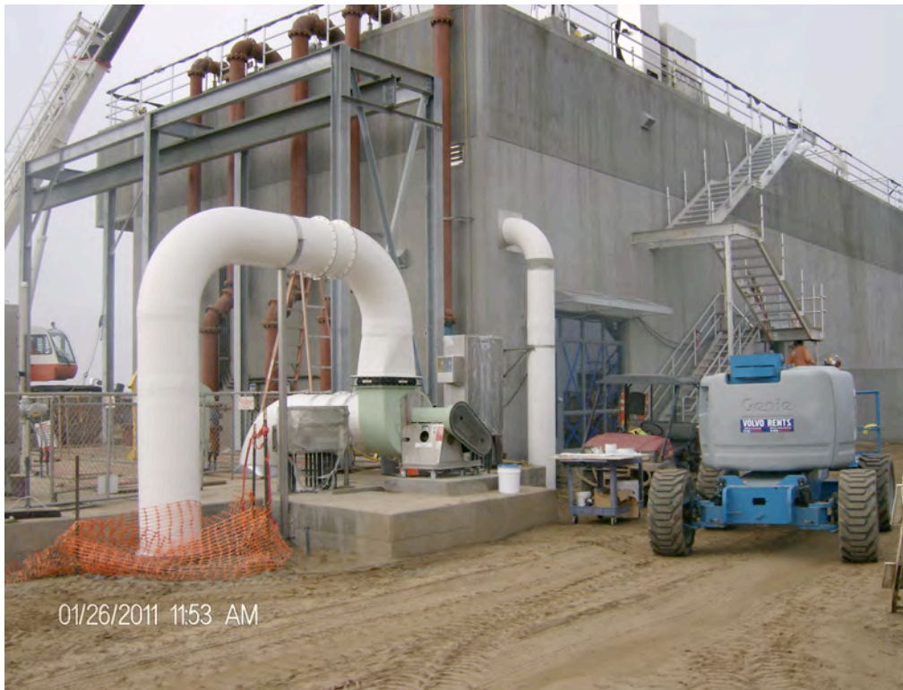
Influent Pump Station Odor Control Fan and Ductwork
