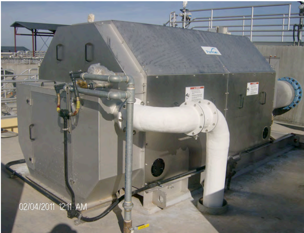
Headworks Drum Screen Ready for Testing
