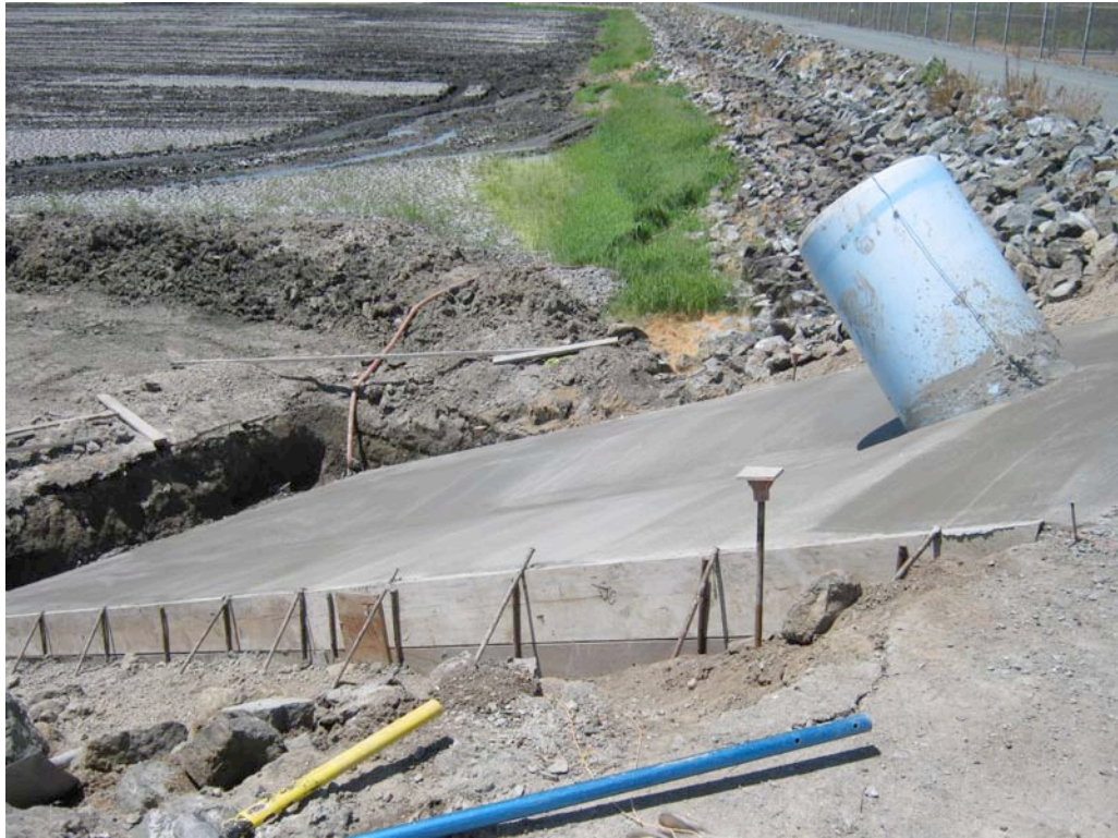
30" Overflow Piping at North Storage Pond
