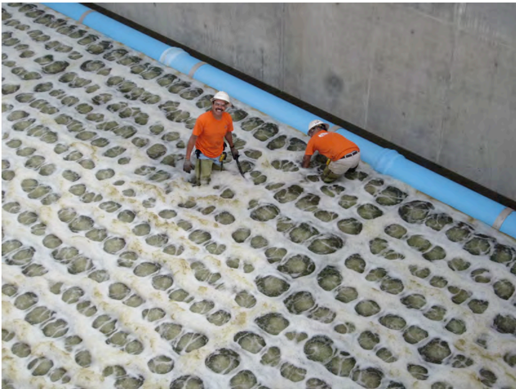
Aeration Basin Diffuser Pattern Test
